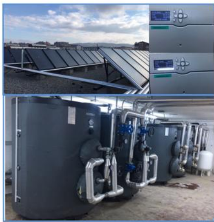
Figure 3 Regional Institute of Public System Installation (collectors, Preheat Tank, Auxiliary Tank, Controller).
